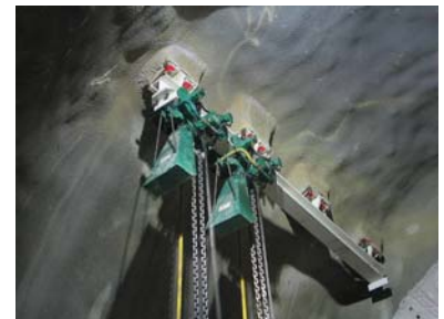
Alp Transit Tunnel: Disassembling works on a tunnel drilling machine with 4 JDN Monorail Air Hoists EH 25.
